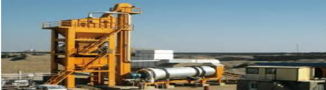
• HOT MIX PLANT
